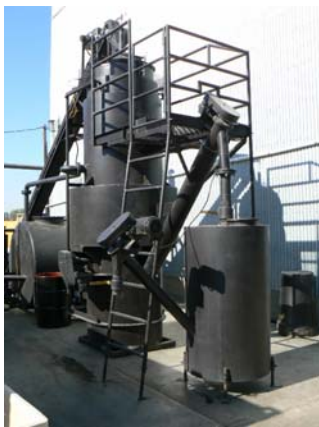
Biomass gasifier in operation at FruitSmart®'s Whitstran facility
